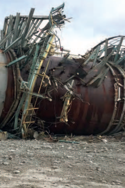
Demolition in progress for d&ri100 new entrant Van Vliet of the Netherlands
