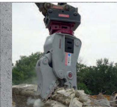
British contractor Cawarden on site at the Becketwell Regeneration project in Derby, United Kingdom
